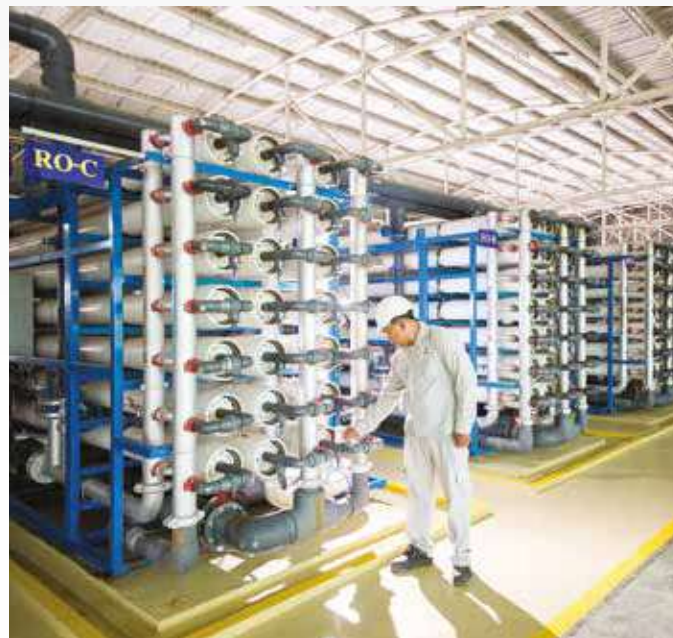
RO membrane system operating at Amata City Industrial Estate, Chonburi, Thailand.
